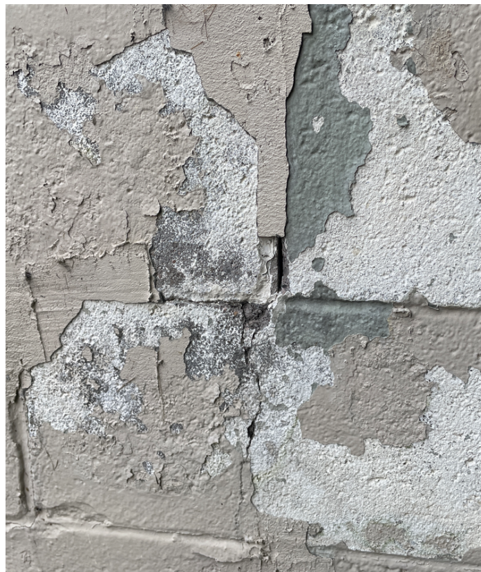
Figure 3: Crack in Block and Missing Joint Mortar
