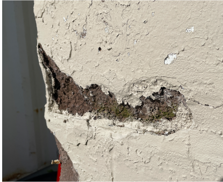
Figure 2: CMU Block Erosion
