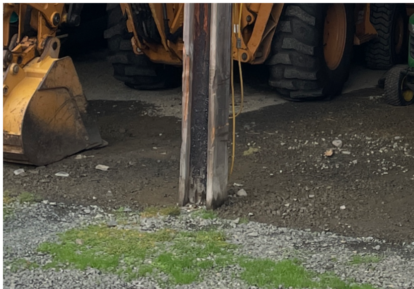
Figure 10: Wood Post in Contact with Grade
