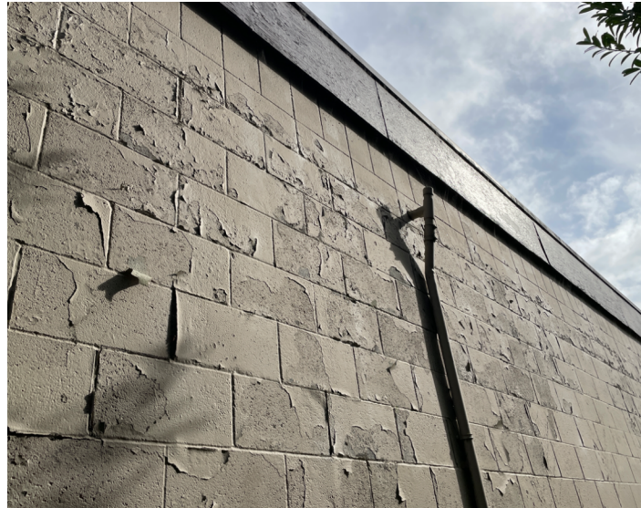
Figure 4: West Wall Peeling Paint
