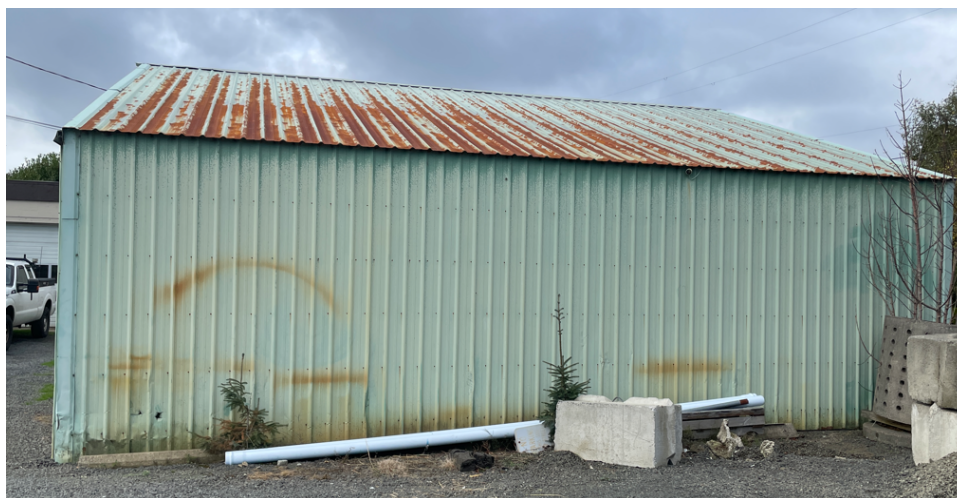
Figure 11: Metal Panel Corrosion
